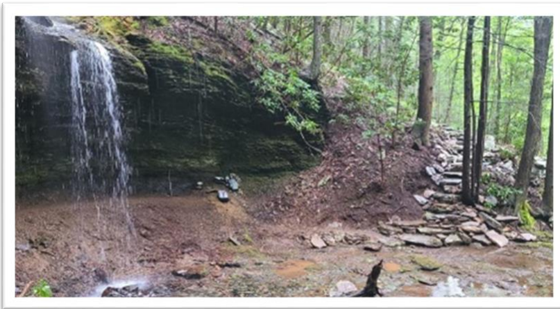
A view from the bottom of the newly constructed staircase on the Lower Piney section of the Cumberland Trail, where the trail continues behind the waterfall.
