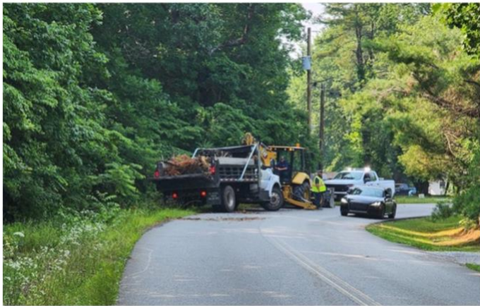
City crews prepare to install a culvert at the site of the Airport trailhead parking lot.
