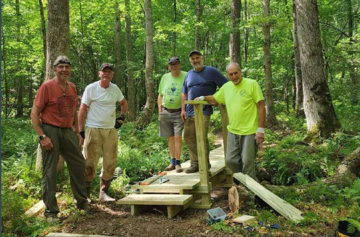
Above: Bridge Building at Airport South Steve Gibbon, Tim Lynch, John Conrad, Dan Coats, Joe Lucas
